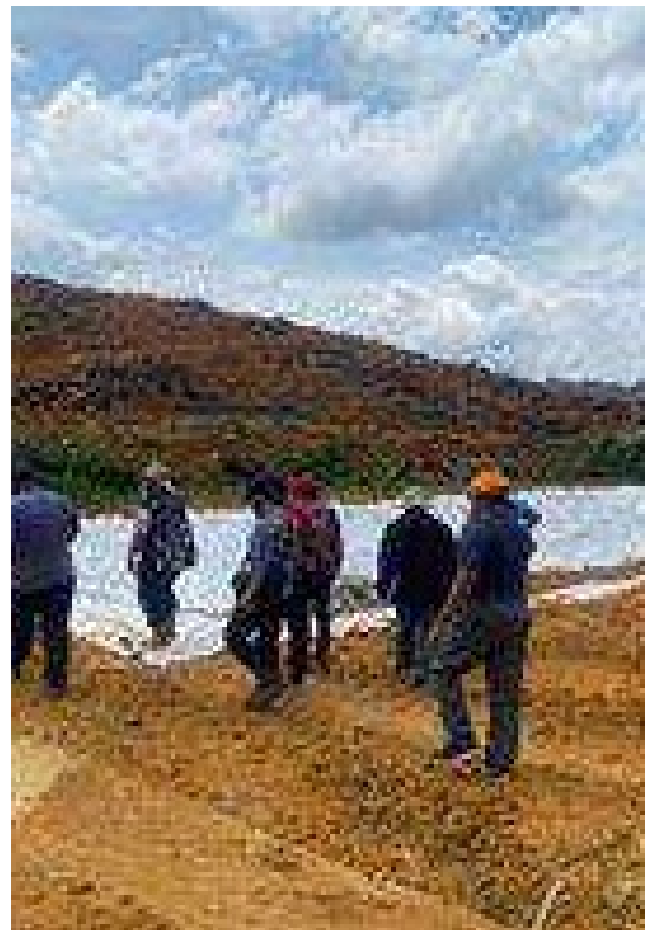
Kolam mendapan ( silt pond ) .
